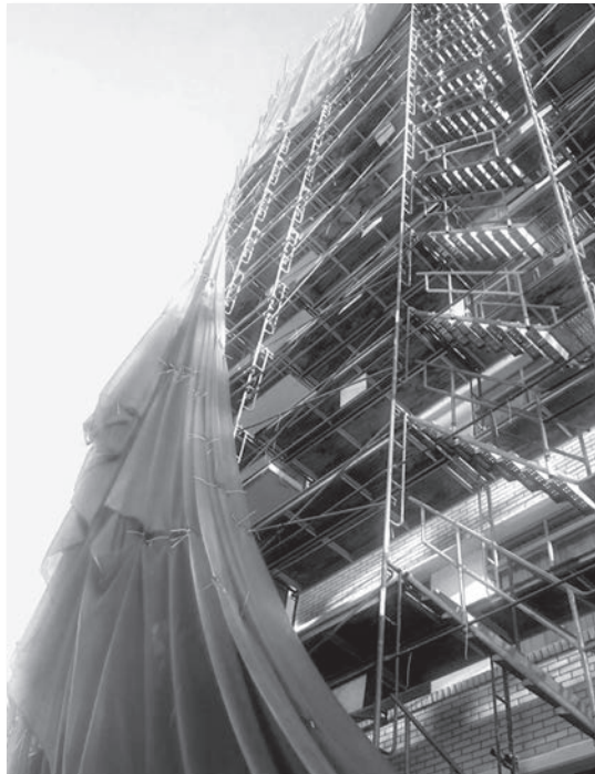
Scaffolding under the tarp at the building on 435 Michigan St., where tenants reported a wide variety of health problems and disturbances due to a years-long renovation project.
